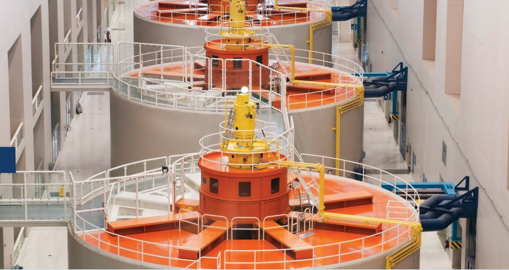
Hydropower generators. © leezsnow/iStock.
