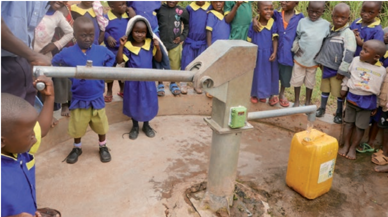
Photo 5.1 SweetSense Inc. Water Pump Sensors Installed in Western Kenya
