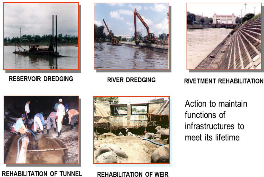
Figure 14 – Water resources infrastructure management
