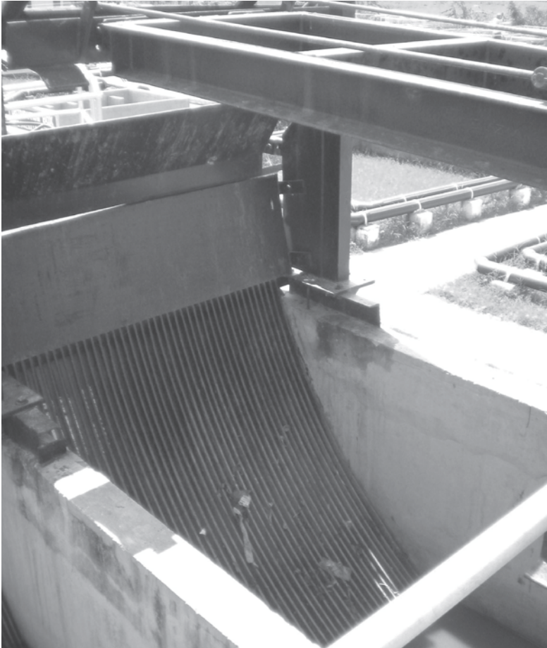
Photo 6.6 Curved screen with rotating raking mechanism
