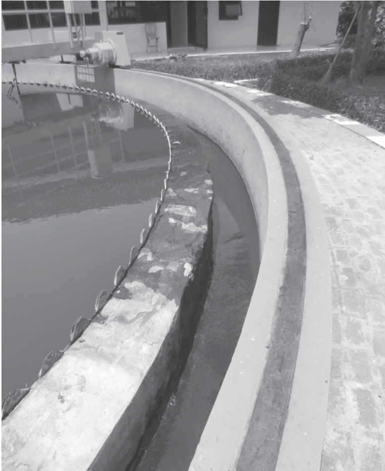
Photo 5.5 Unbalanced flow resulting from poorly levelled weir
