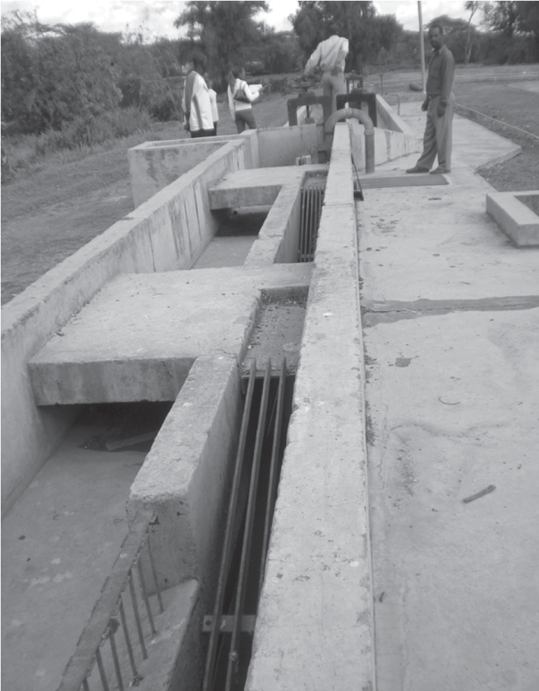
Photo 5.3 Inclined screen with operator access
