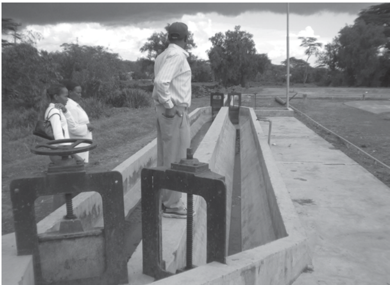
Photo 6.9 Grit channel at wastewater treatment plant, Naivasha, Kenya
