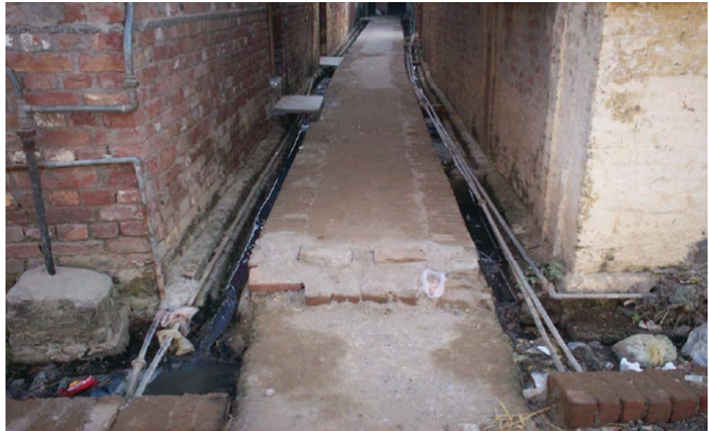
Image 3.1: Water Pipelines Inside Open Sewerage Drains
