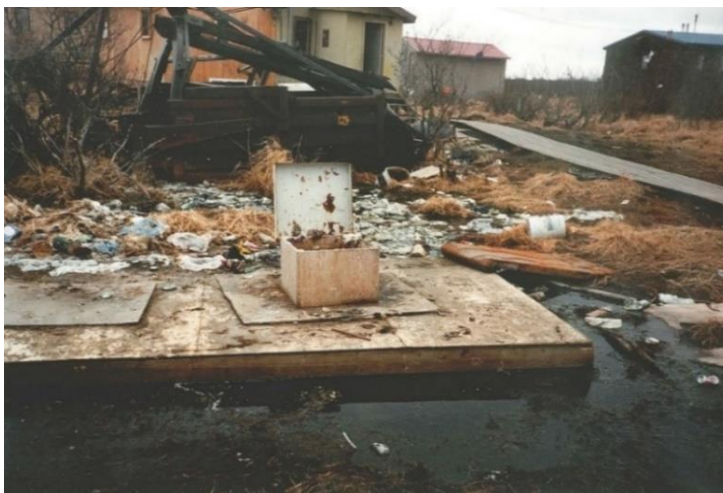
Photo A1-1: Underground Communal Waste Tank, Alaska
