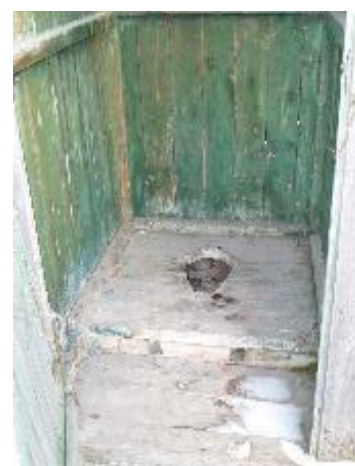
Photo 4-2: Pit latrine with slab, Kyrgyz Republic
