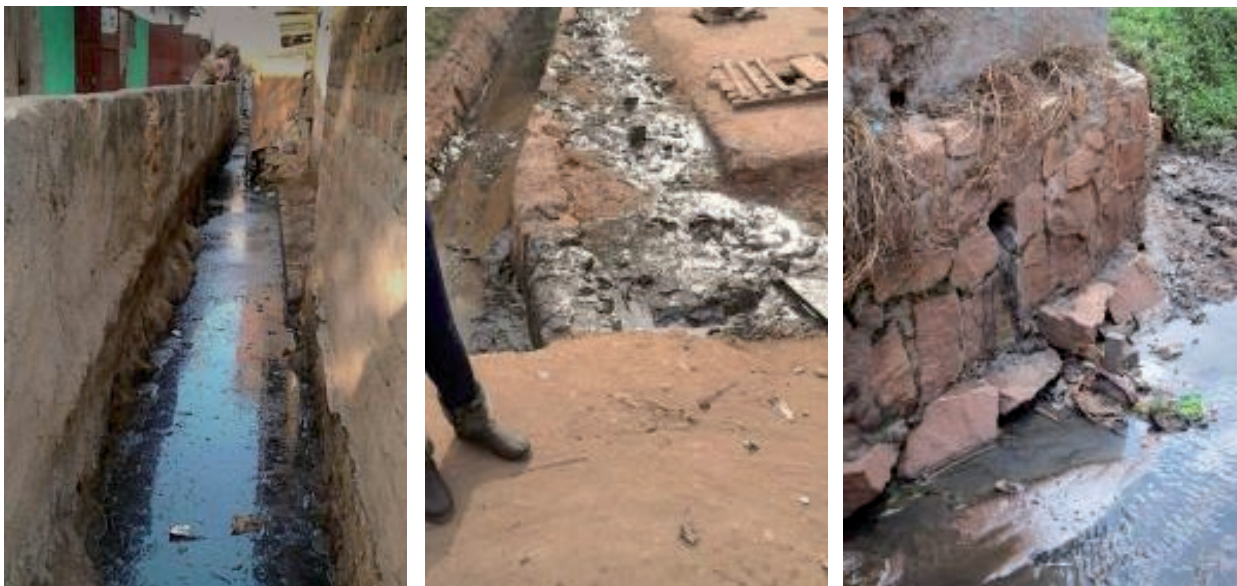
Sludge discharged directly to drainage channels in Kampala. These pictures were taken in several locations and are representative of any of a growing number of towns, notably Mukono, Wakiso, and Masaka.
