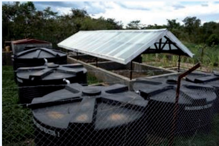
A small sludge treatment plant developed by an NGO, Water for People, outside Lira.
