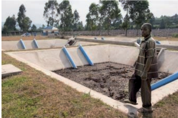
The new sludge drying beds in Ntungamo, dedicated to fecal sludge deliveries.
